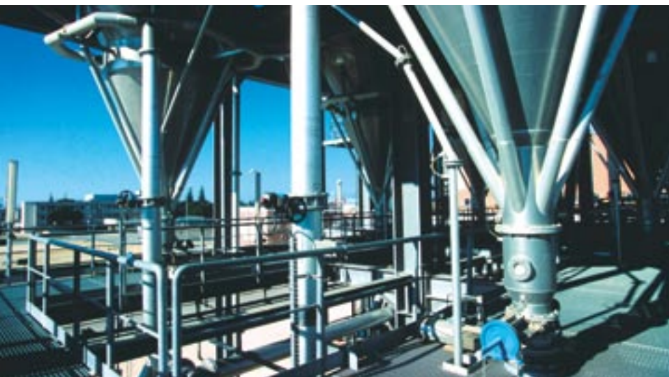
Blending pipes and blending chamber of a Zeppelin Multi-Pipe Blender with integrated aeration ring for degassing on the left
